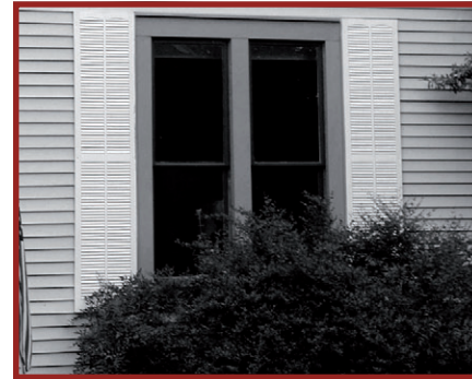
5.5 Note how these shutters do not relate to the size of the window opening and that they clearly appear to be inoperable.
