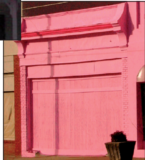
Colors that are visually incompatible with the historic character of the district, such as hot pink, are not recommended.
