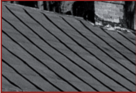
Figure 4.2 Note how the ridge and eave details on this traditional standing seam metal roof have been folded down and how the pattern created results in a softer visual character.
