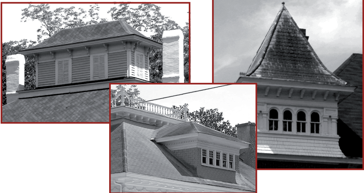
Example A (top left). This is an example of a ventilation cupola. Example B (bottom center). Note how the the “widow’s walk” and dormer are character-defining features of this roof. Example C (top right). This tower visually dominates the corner of this house and helps to define its character. All of these features add architectural diversity and interest to the historic district.
